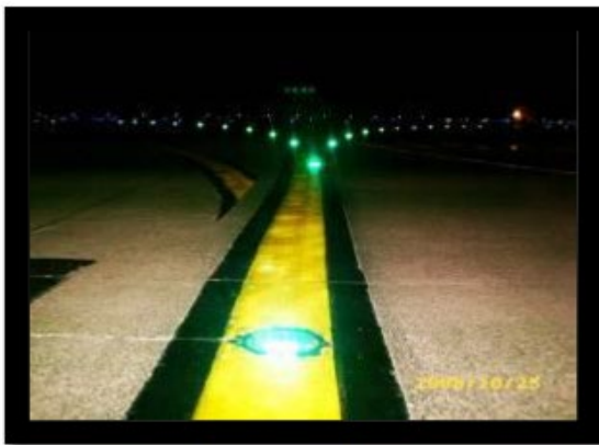
Figure 4.17. Taxiway Centerline Lights.
