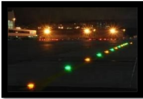
Figure 4.18. (Taxiway Centerline Lead-Off/Lead-In Lights.)
