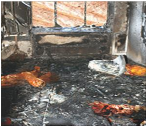
Figure 4.35. Damaged Building Interior with Remains.
