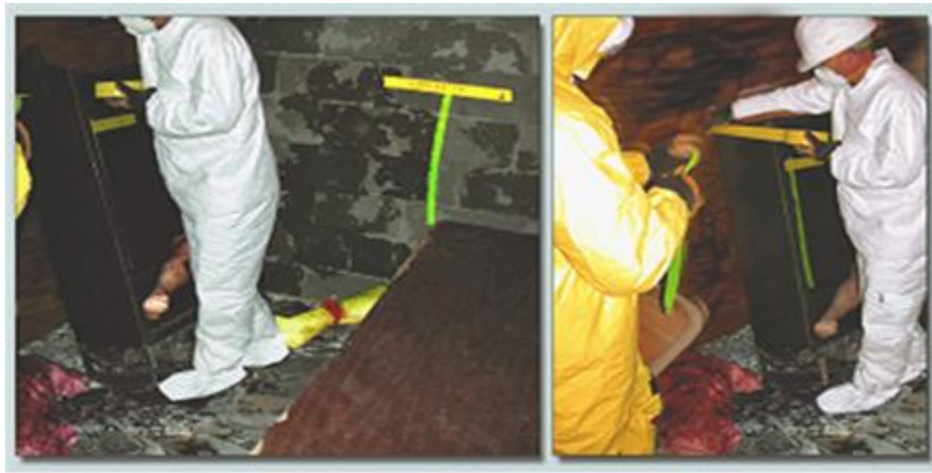
Figure 4.36. Damaged Building Interior and Marking Methods.
